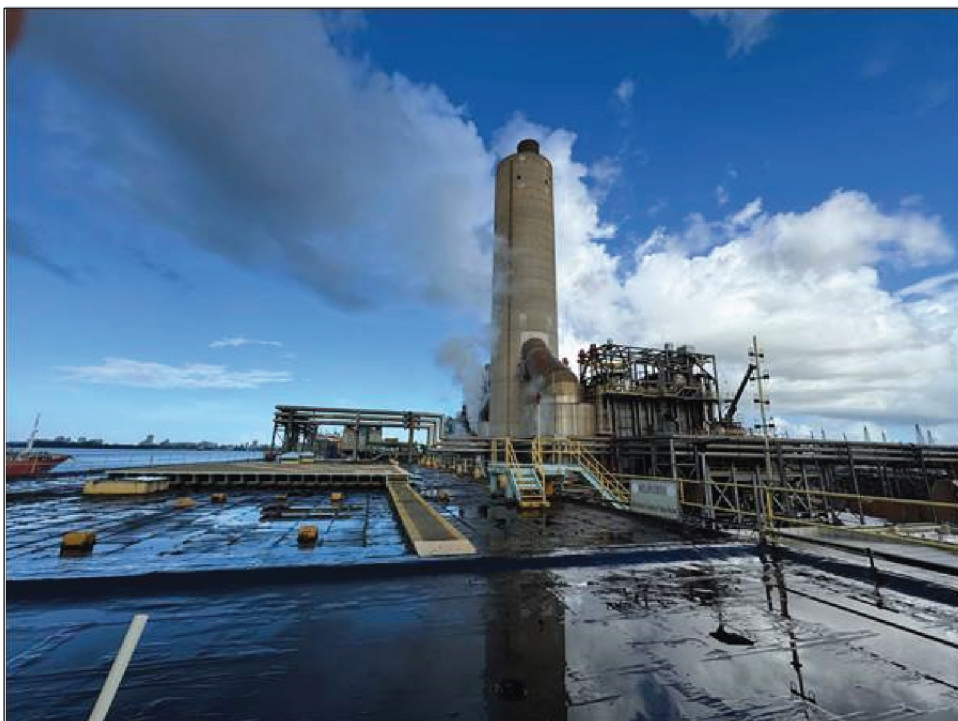
Figure 3: Federal Emergency Management Agency Public Assistance Project Eligible to Receive Community Development Block Grant Funds to Help Cover Cost Share: San Juan Central Generation Station
